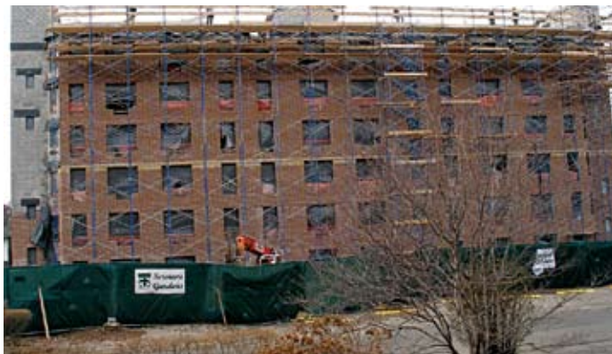
Serviam Gardens construction progress on the Bedford Park property (photo by Marcia Kimball, o.s.u.)
